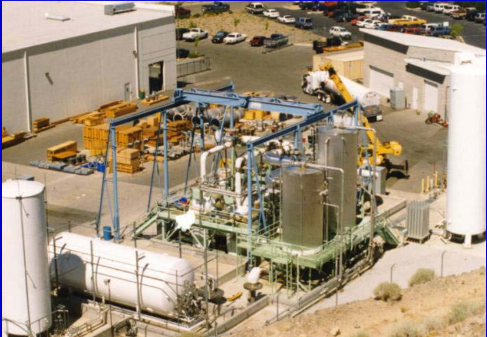
Ebara LNG Test Facility in Nevada
